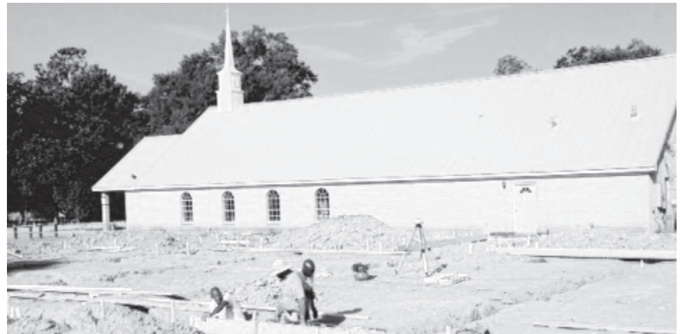
Mt. Carmel Baptist Church constructs new fellowship hall (Photos by Susie A. Wolfe)
